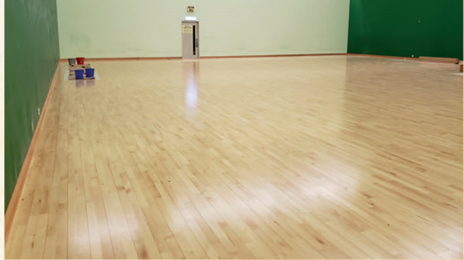
Replacement of the Juncker hardwood floor for the Badminton Hall 更換羽毛球場的實木地板
